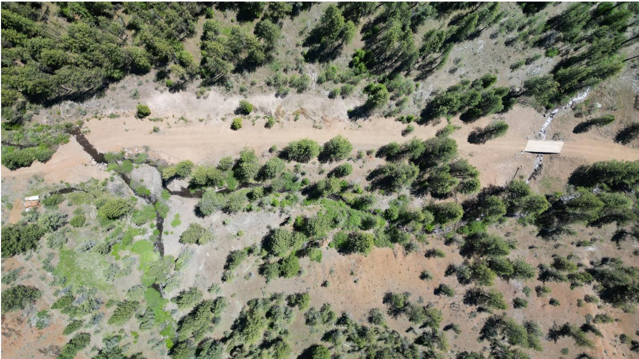
Aerial view of Dutchman Creek Bridge and new confluence with Big Log Creek, and the Foley Culverts that were Removed – June 12, 2024
