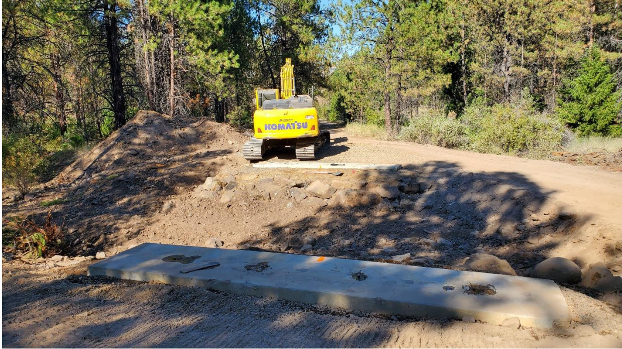
Bridge abutments place at Dutchman Creek Crossing prior to bridge stringers – August 18, 2023
