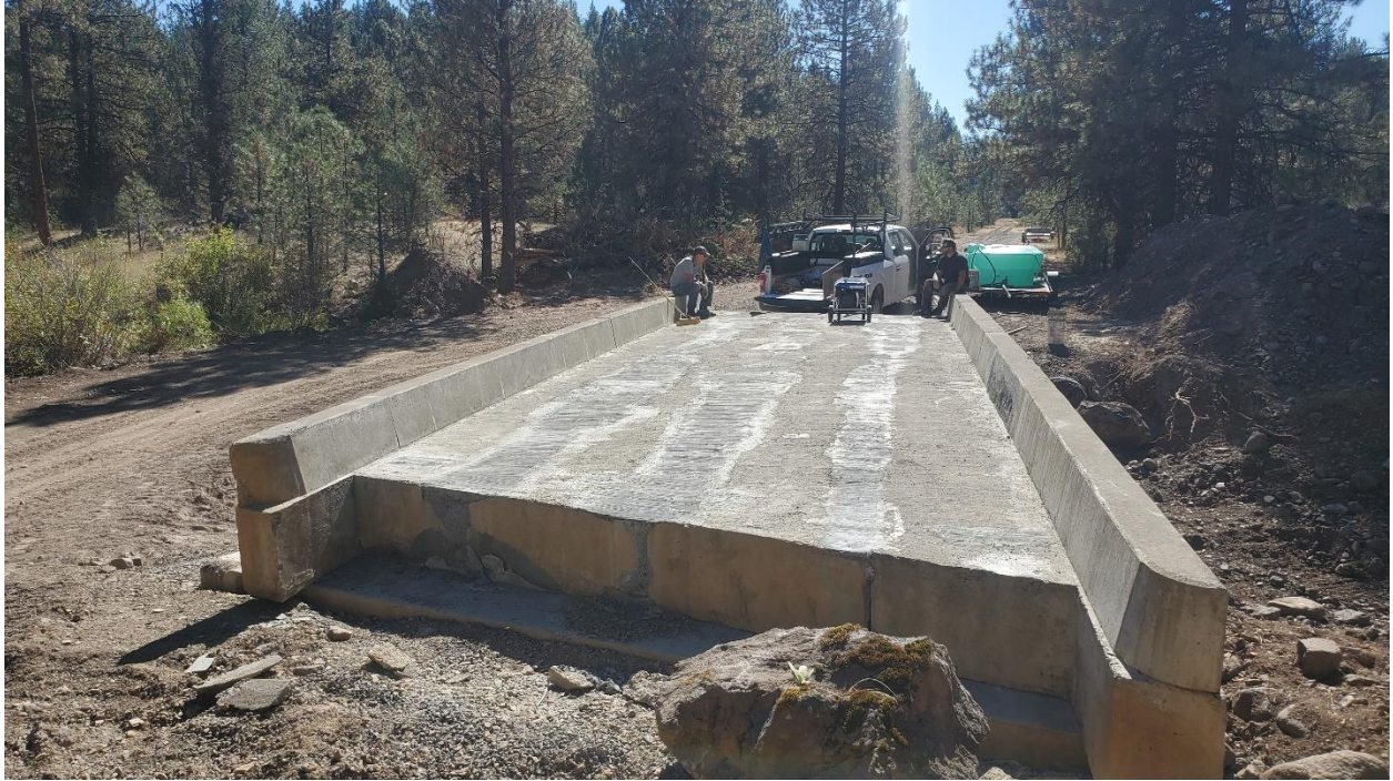
Grout work done, ready for backfill/road construction and temporary road removal – September 9, 2023
